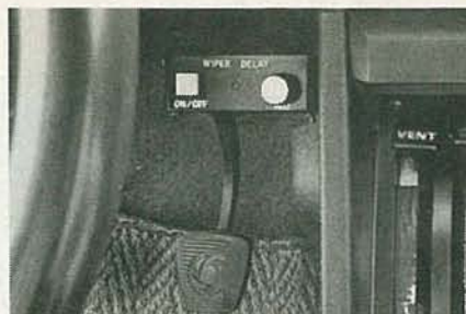
FIG. 5—THE INSTALLED SOLID-STATE WIPER CONTROL under the dash. Here, the holes for the lid were drilled out, and 4-40 screws were used to mount the case under the dash. You can also use the lid, and attach the case with Velcro or double-sided tape.
